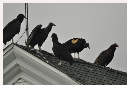
Damage to buildings
